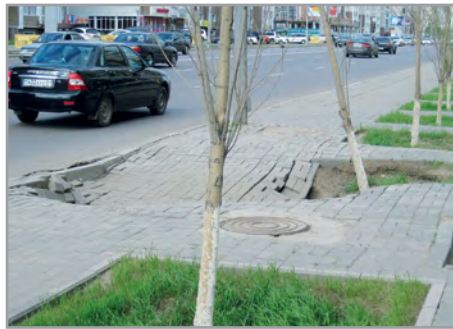
Subsidence in urban area induced by water network leakage. Credits: meadowsaffron on flickr
